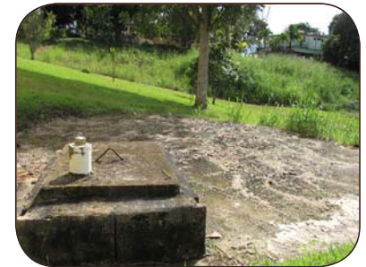
Keep septic tanks sealed.
